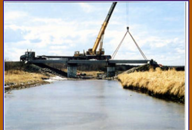
7-12 Erecting third span girders on top of previously erected middle span girders
